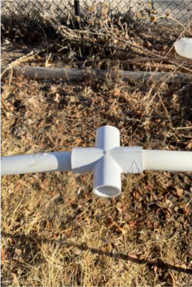
Step 5 - Use the cross fitting Charlotte pipe to connect the two PVC pipes in the middle of the bed to form the middle arch. You should now have 3 arches.
