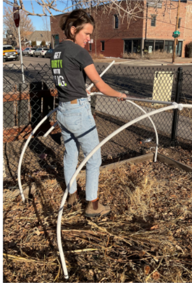
Step 6 - Connect the arches with the 3/4" PVC pipes and the "T" Charlottes to form a stable structure.
